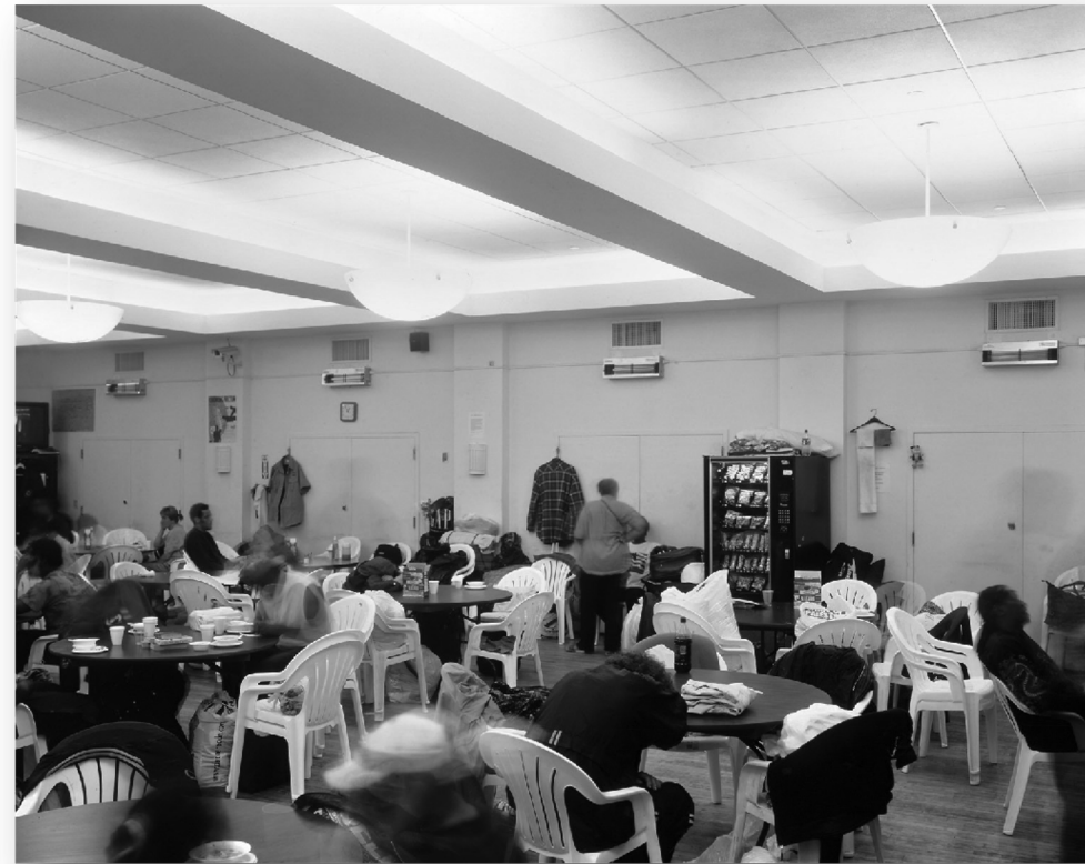
Tuberculosis Ultraviolet Shelter Study New York City shelter in a church basement. Note the ultraviolet germicidal irradiation fixtures located on the upper wall, directly below the vents. Photo: ©Randall Perry Photography.
